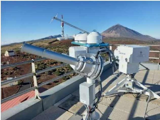
Figure 10.3. The EKO MS-711 spectroradiometer installed at IZO.
