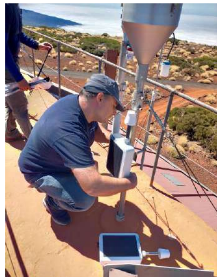
Figure 17.10. Installation of new PM-LCS (four sensors) at IARC for the CREWS project.
