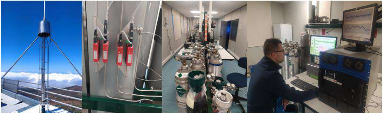
Figure 20.3. Ambient air/gas standard plumbing diagram of the Izaña-ICOS station. At the bottom, from left to right, photographs showing parts of the installation: sampling, flow meters, gas tanks and work station next to the instruments.
